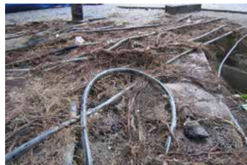
Roots and cables compete for space underground.
