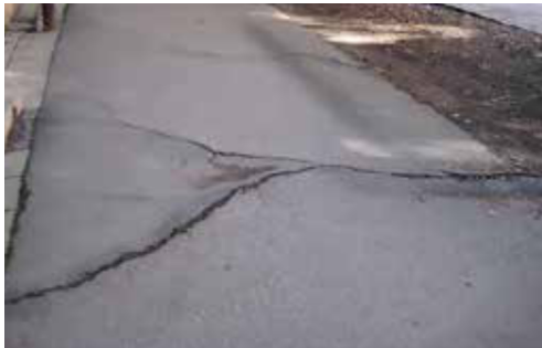
Damage to city surfaces caused by roots.
